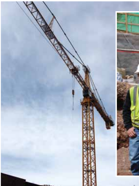
The electric crane is used to lift and move a variety of objects from one location to another on the construction site.
