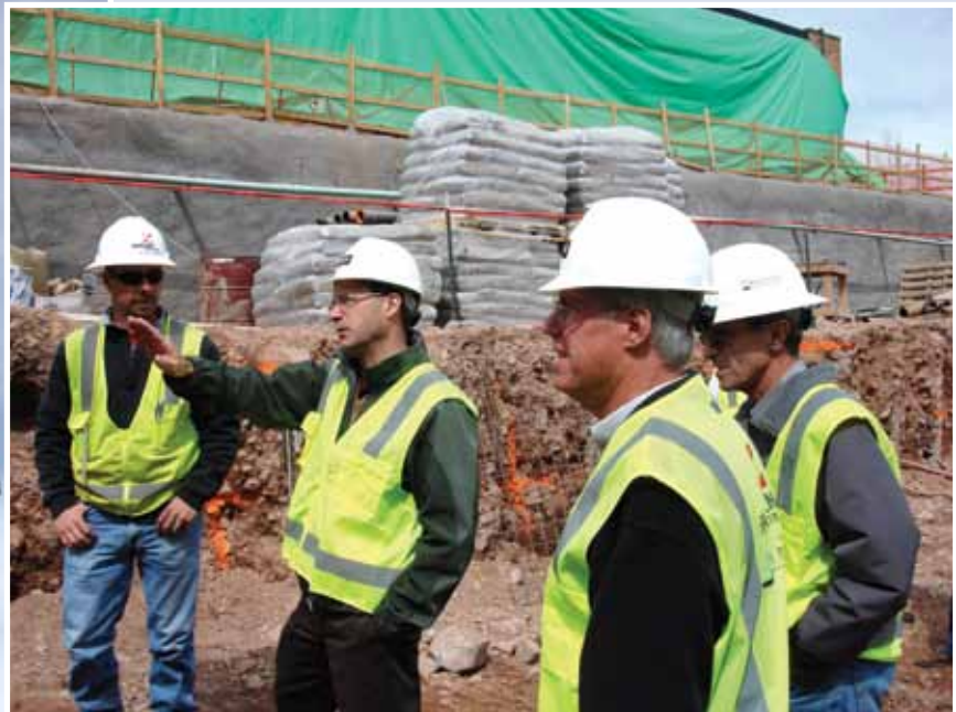
Haselden supervisor Chance Warren conducts a site tour for Aspen Valley Hospital CEO Dave Ressler, CFO Terry Collins, and community liaison Frank Goldsmith.
