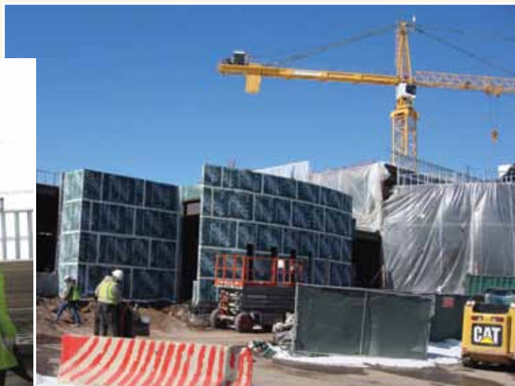
The front entry of Phase II and the new cafeteria (left) begin to take form.
