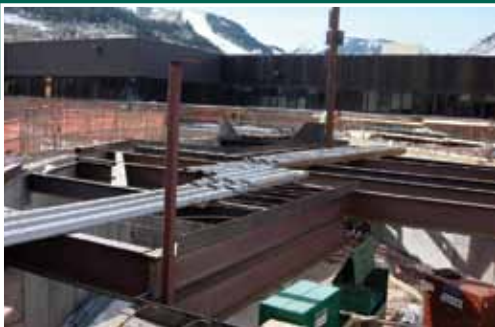
Structural steel that will form the expansion of the patient care unit was placed in the fall of 2011.
